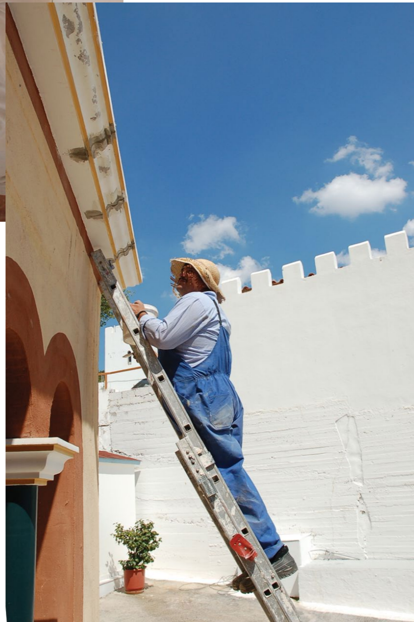
...and also on the exterior—ten years have wrought wear and tear, which require maintenance.
